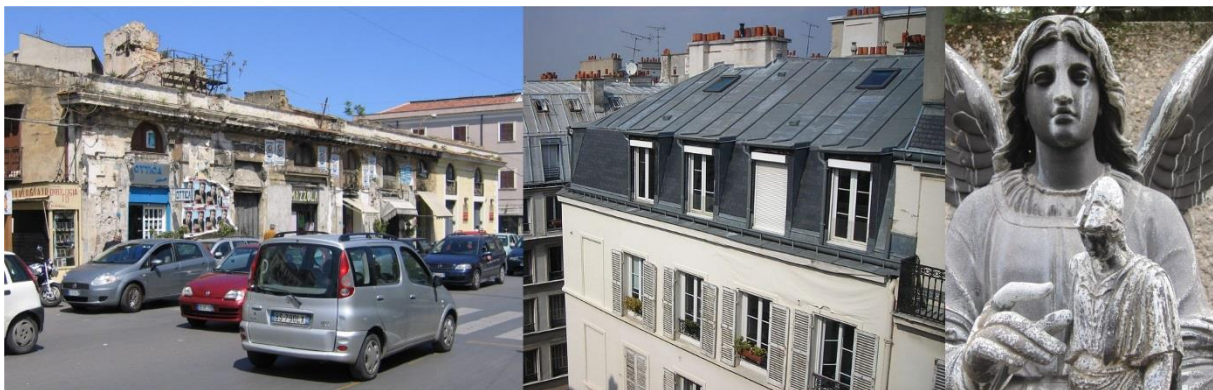
Figure 2: Weathering of a limestone facade in Palermo, Italy, of zinc roofs in Paris, France (Wikipedia), and of a zinc monument (19 th century, from a German workshop) in Oslo, Norway.
