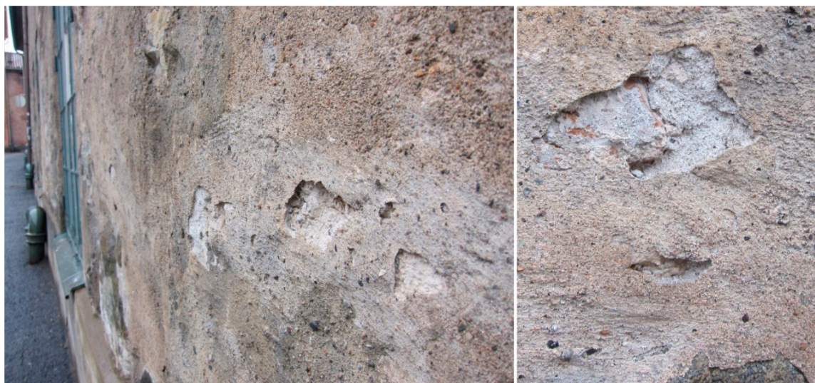
Figure 3. Initial and probably accelerating deterioration of a rough sand-containing rendering applied on the uneven surface of the building seen in Figure 4d, with protruding parts of stones from the wall under the rendering.
