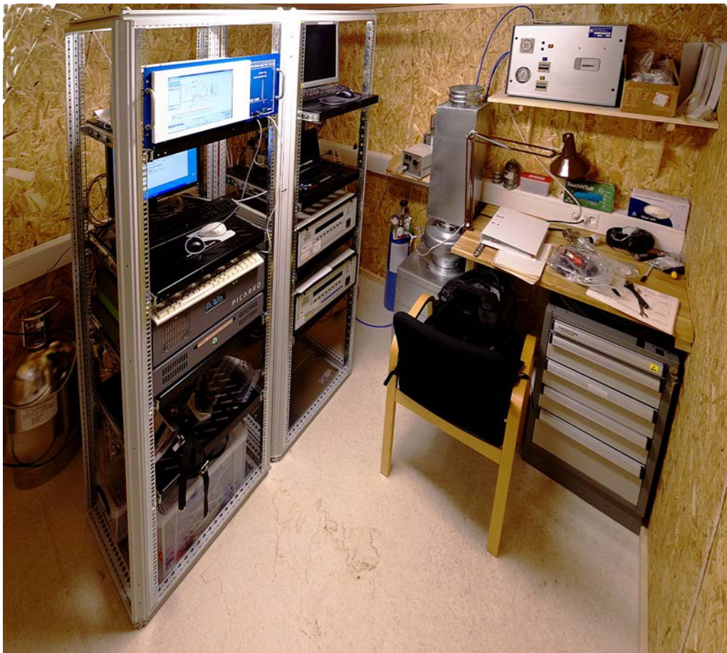
Figure 1: Interior of the measurement station Transformatorbua with instruments and other necessary equipment. (Photo: Ove Hermansen, NILU).
