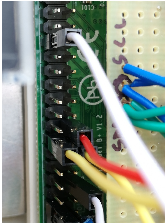
Figure S1.3. A detail of the wiring between the acquisition board and T&RH sensors to the GPIO of the Raspberry Pi. Here are shown the GPIO pins from 9 (GND with white wire on bootom-right of the pic) to 30 (GND with white wire on top-left of the pic).
