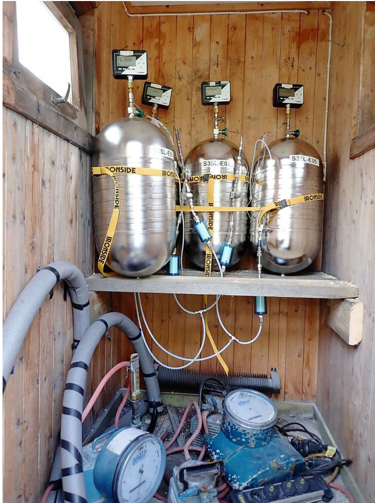
Figure 4: One inlet line from each of the chimneys was split to both CSIRO and NILU restrictor
